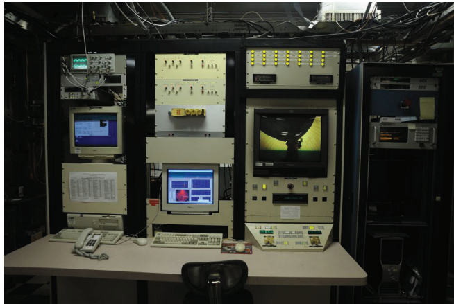
The primary control for the Westford 60' antenna.
