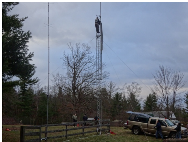
The bottom part went up one section at a time, with a gin pole.
