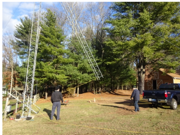
The fold-over portion was assembled from the ground, from the back of a pickup.
