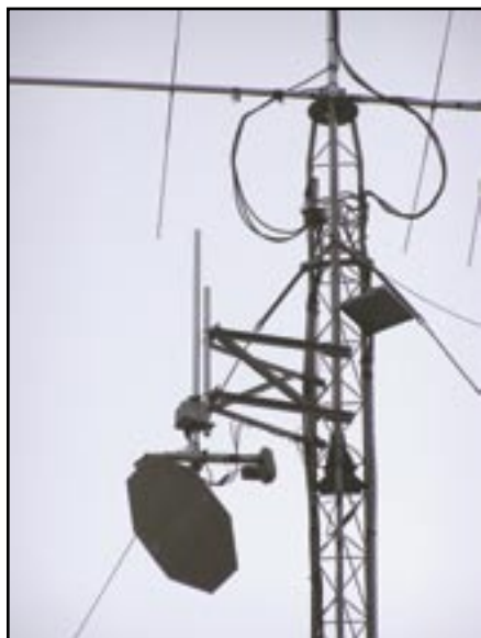
Figure 3 — Flyswatter side-mounted on tower.
